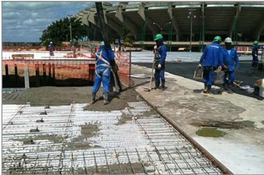
Application of PENETRON ADMIX-treated concrete on Castelão. Construction joints have already been prepared with PENEBAR SW-55.
