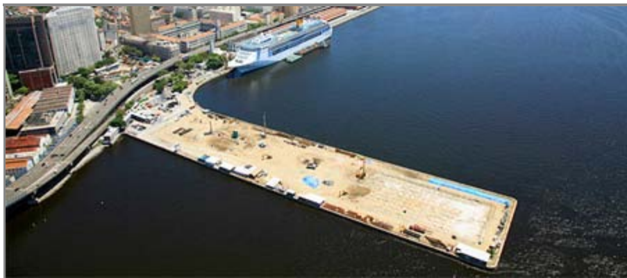
Construction site of the Museum of Tomorrow; concrete slab was treated with PENETRON ADMIX and PENEBAR SW-55.
