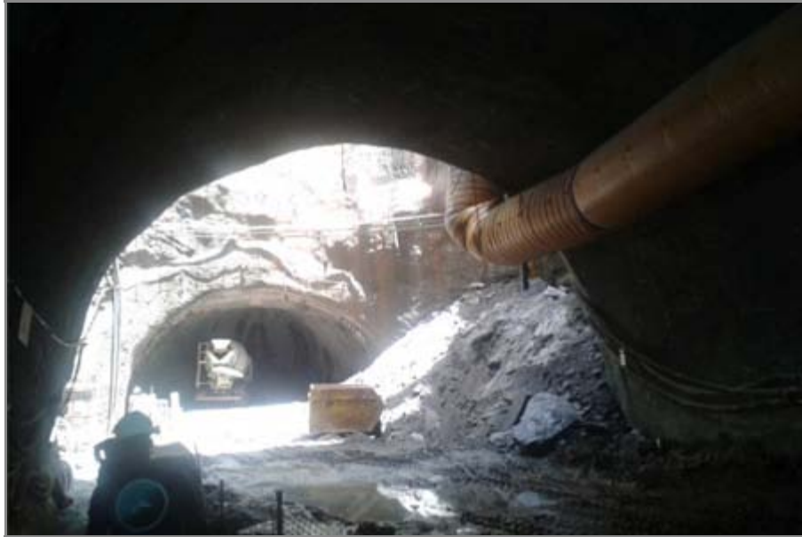
Tunnel excavation near the port; PENETRON ADMIX is used in the shotcrete.
