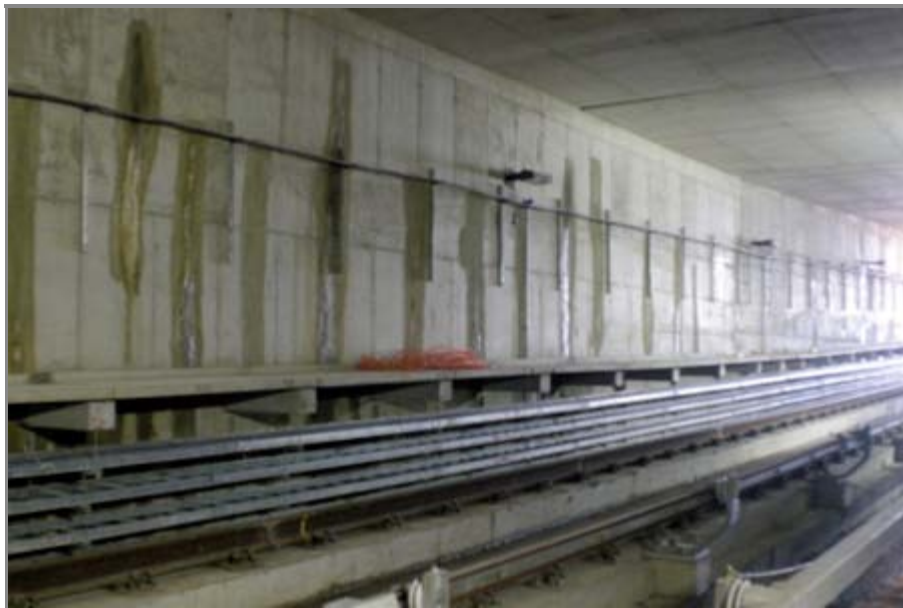
View of the cracks before the PENETRON treatment.
